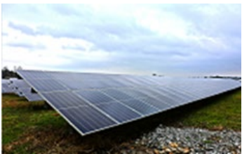
Brighter Future Solar Power Generation
