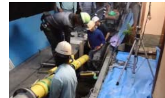
Solving ageing pipe issues
