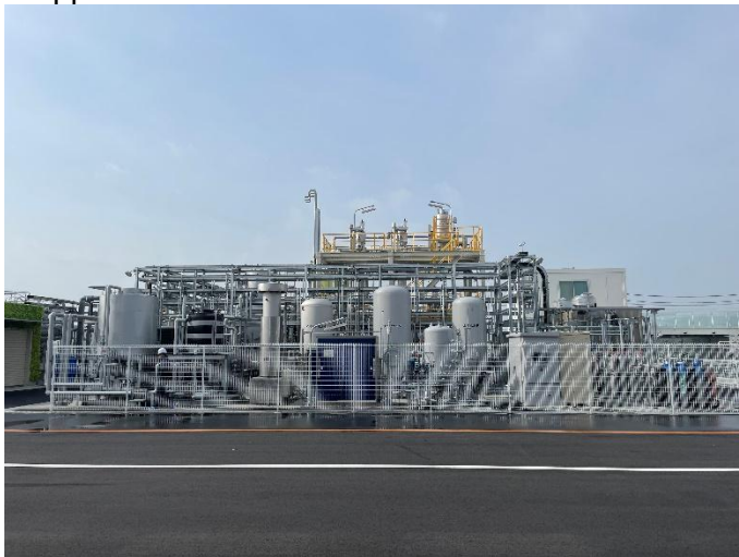
■ Appearance of Bakeru LABO
