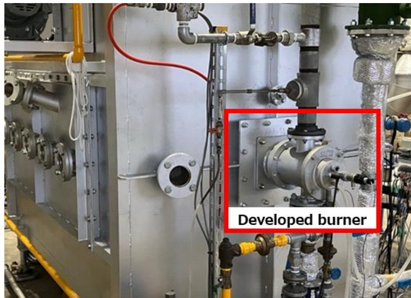
Photo of the heat exchanger-equipped exhaust heat recovery burner installed in a test furnace at a Daigas Energy experimental facility
