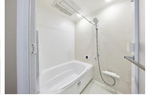
⑥ Energy conservation equipment (water-saving bathtub/shower/faucet)
