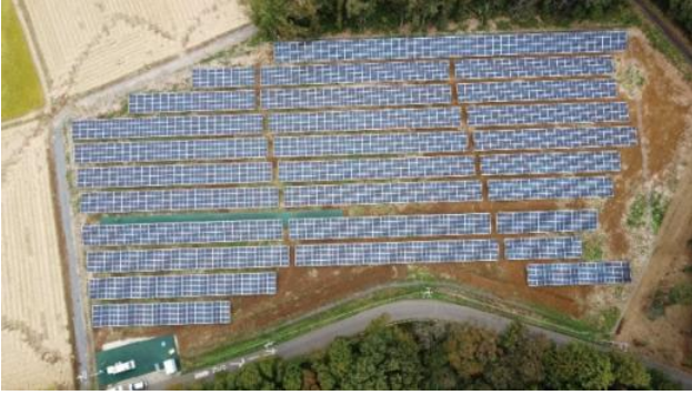
Solar power plant in Ibaraki Town, Ibaraki Prefecture (Installed capacity: 1,050 kW)
