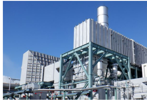
Full shot of the high-efficiency gas turbine
