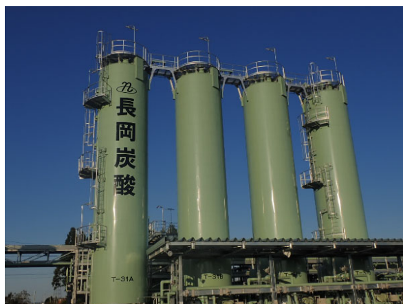
[Liquefied carbon dioxide production plant]
