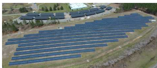
Solar power plant developed and constructed by SolAmerica Energy
