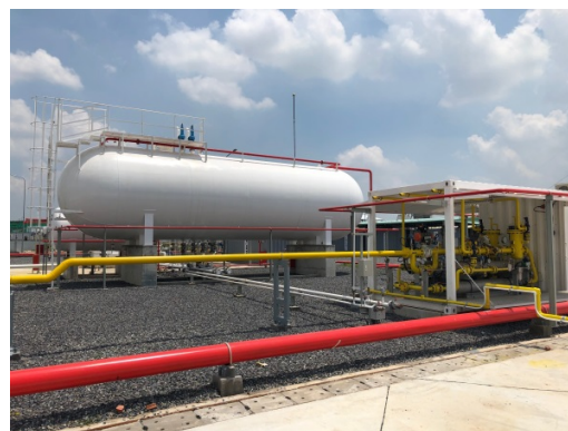
External appearance of the gas supply facility at the Phu My 3 Specialized Industrial Park.
