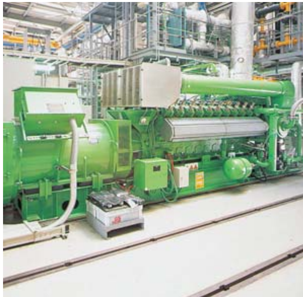
gas cogeneration system
