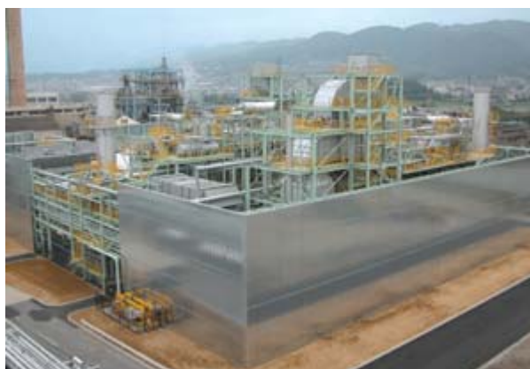
"power source cogeneration system" constructed within the premises of the Uji Plant of Unitika Ltd.
