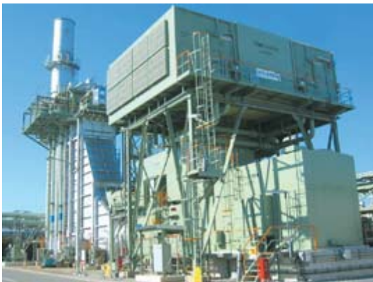
Electric power generation facilities at the Himeji Terminal
