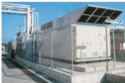
Cogeneration system using biogas
