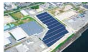
Torishima Solar Power Plant
