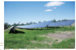
Aurora Solar Power Generation Project
