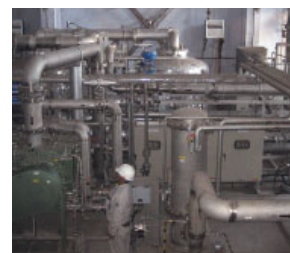
Low-concentration CMM (coal mine methane) enrichment equipment (verified)
