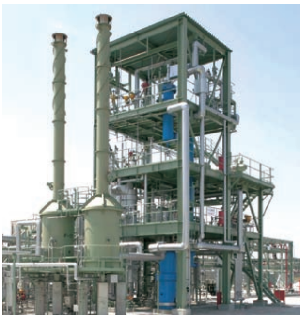
A-ATG Pilot Equipment (verified)
