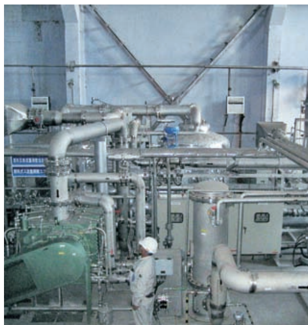
Low-concentration CMM (coal mine methane) enrichment equipment (verified)
