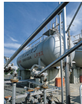
LPG Recharging Station
