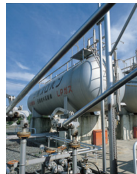
LPG Recharging Station
