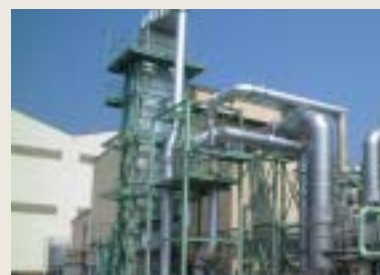
OMviro demonstration plant using a smoke emission treatment catalyst
