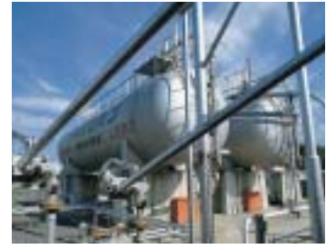
LPG recharging station operated by Nissho Iwai Petroleum Gas Group
