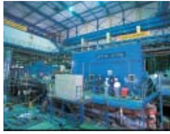
This 150-MW power generator began operations in April 2003 at the Torishima Energy Center (Osaka).
