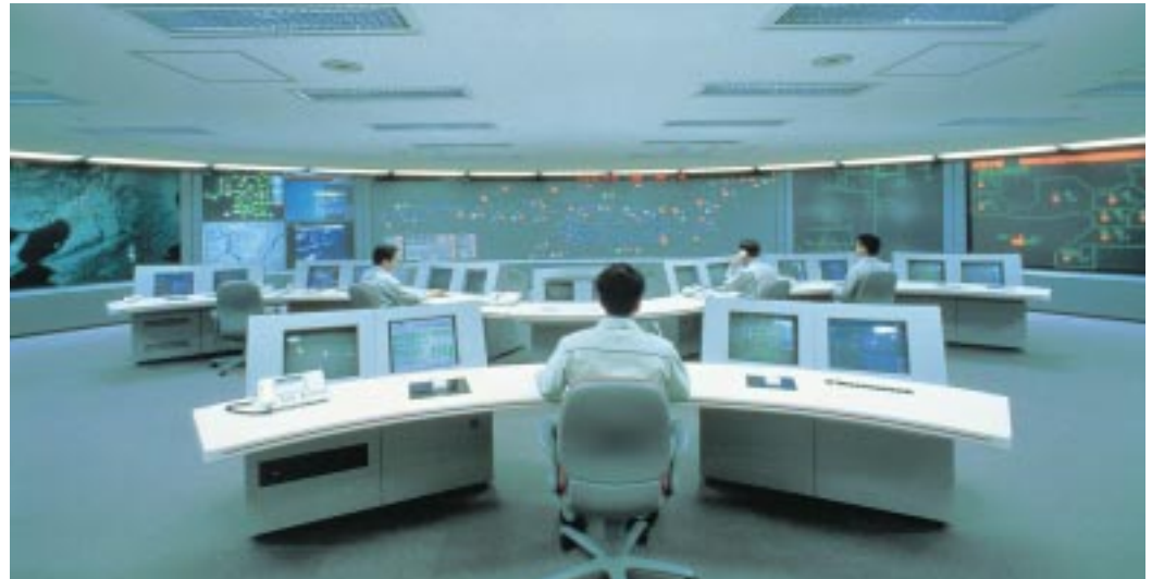
The Distribution Control Center monitors safety of supply systems.
