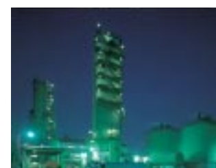
An air-liquid separation facility (CRYO-AIR)
