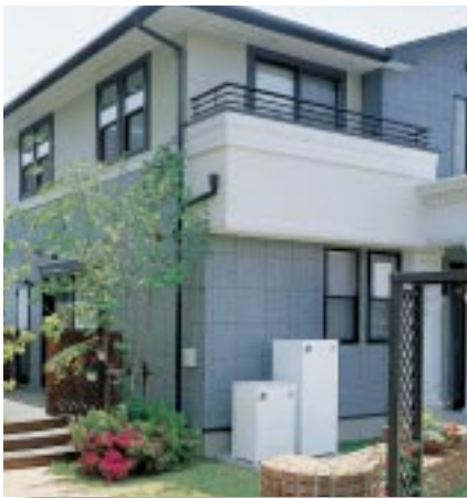
Residential Fuel Cell Systems under performance monitoring
