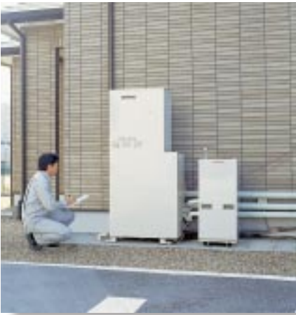
Field Testing for 1kW gas engine cogeneration system
