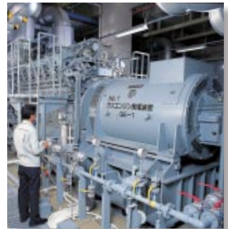
Gas Engine Co-generation System
