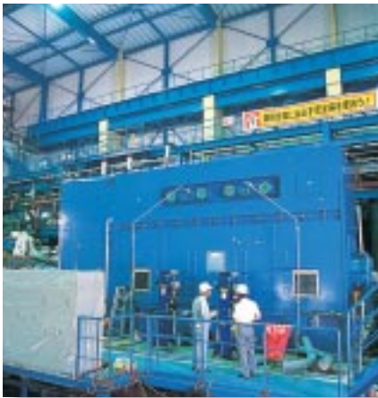
IPP facility in The Torishima Energy Center
