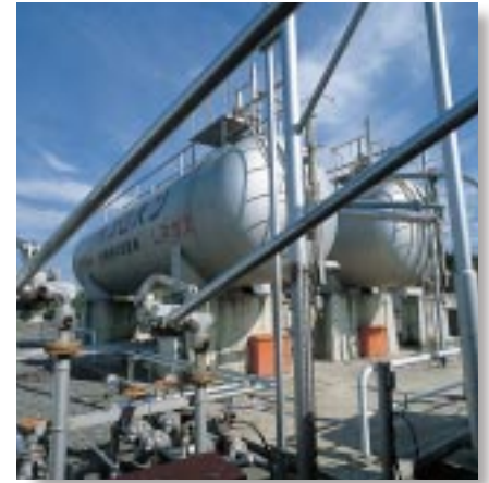
An LPG replenishing facility (Nissho Iwai Petroleum Gas Group)
